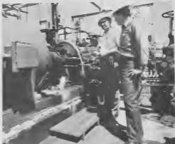
The camera catches Vicente here at the Gasoline Pumphouse just as he detects a leaking pump. Operations Supervisor Coby Geerman witnesses Vicente's immediate action as he writes out a report. E camera ta captura Vicente aki na Gasoline Pumphouse net ora el a descubri un pomp ta lek. Operetione Supervisor Coby Geerman ta testigo di Vicente su accion inmediato mientras el ta escribi un rapport.
